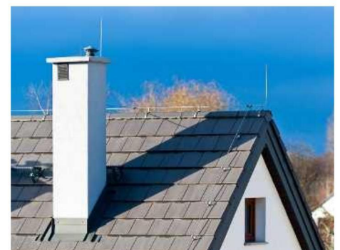
Fig. 15 External lightning protection, here on a private residence, for example
